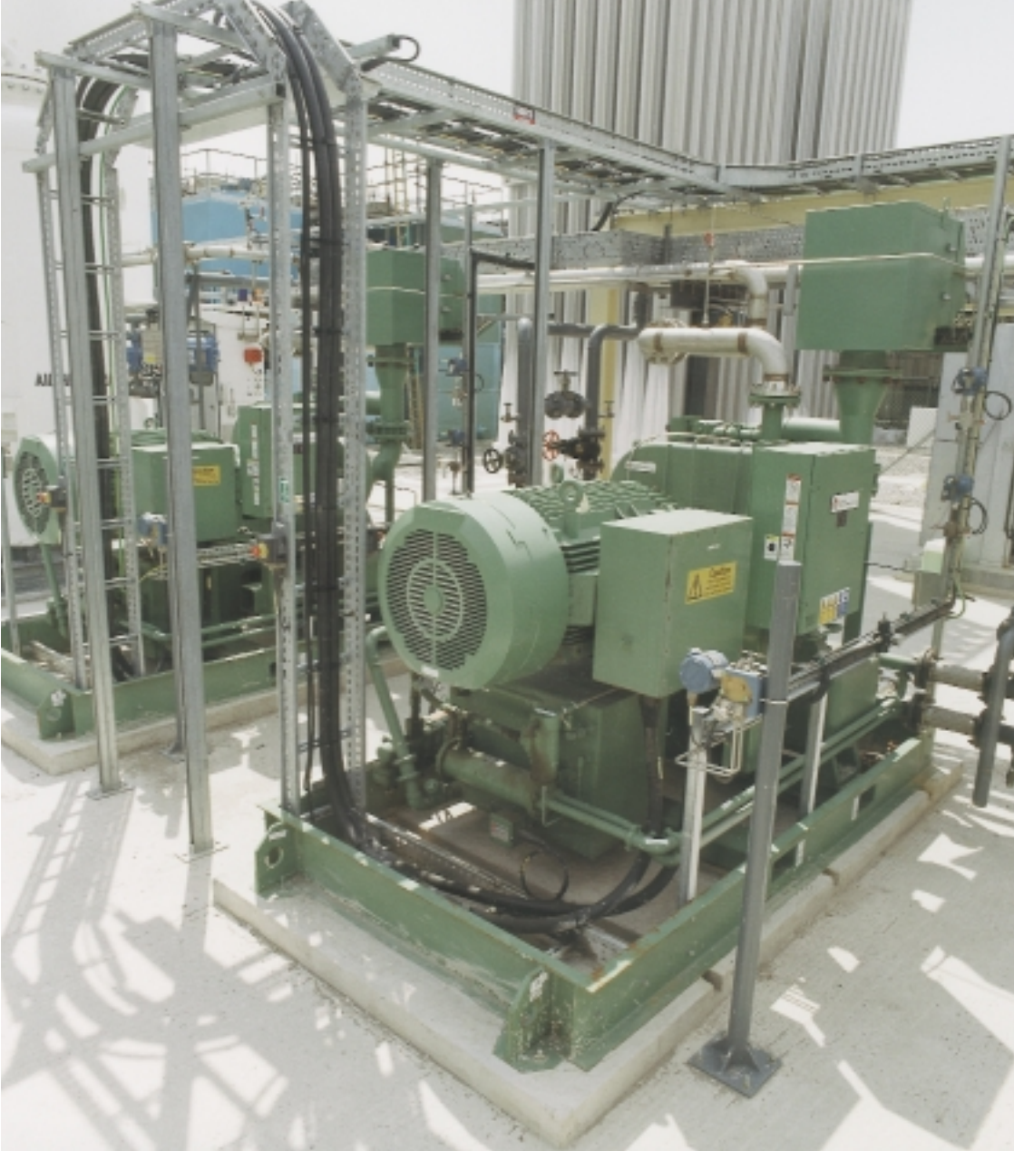
Air Products' tailored compressor supply solution for AstraZeneca
